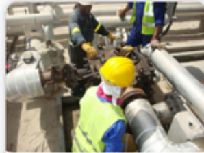
PREVENTIVE PLANT MAINTENANCE & INSPECTION
