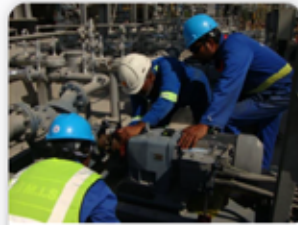
PUMP INSPECTION & MAINTENANCE
